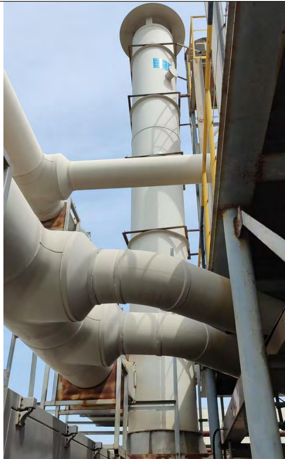
1#车间废气排气筒 DA002
